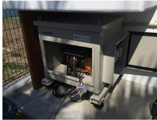
Fig. 10 Electric Transforming unit from Ship-to-Land
