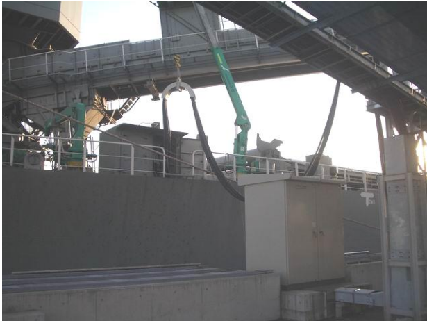
Fig.5 Electric power supply from land to ship
