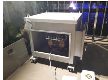
Fig.12 Electric transforming unit from ship to land
